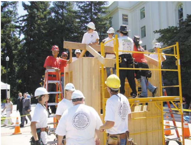
Golden Sierra High School students from the Ultimate Cutting Edge Construction Team constructing a building on the State Capitol lawn.
