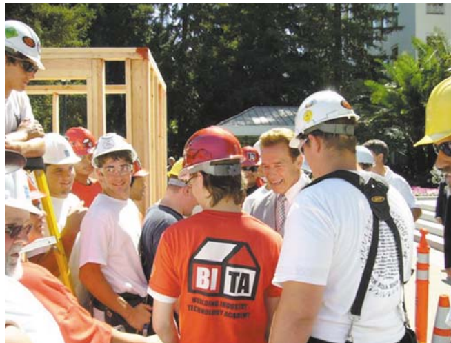
Golden Sierra High School students from the Ultimate Cutting Edge Construction Team meeting Governor Schwarzenegger while constructing a building on the State Capitol lawn.
